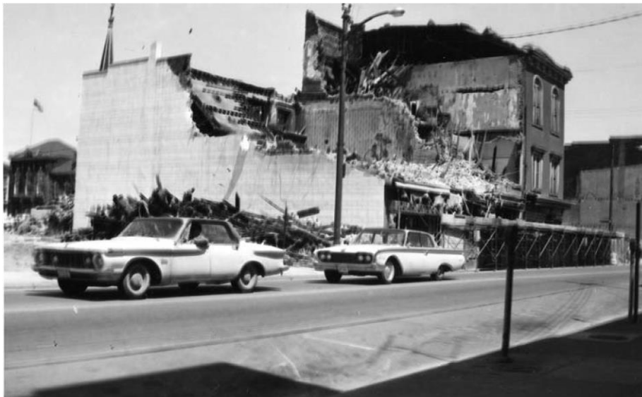
Destruction of Rosenberg Department Store in 1965 as part of the Gadsby Urban Renewal Project ( Special Collections, Alexandria Library )
