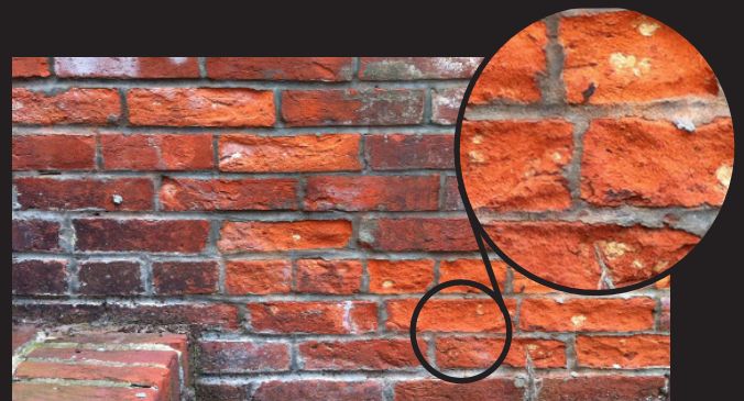
In this example, repointing with a Portland cement mortar has irreversibly damaged the historic brick, causing spalling. Spalling is when the hard-fired face of the brick breaks off due to an impermeable mortar joint.
